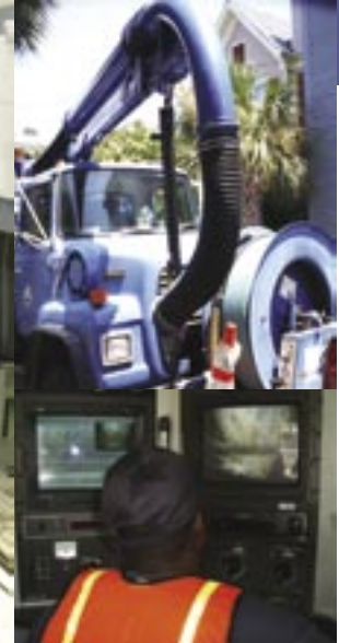
Vactor truck (top). Inspecting a sewer line using a remote-controlled video camera (bottom).
