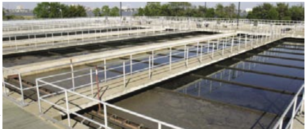
Secondary clarifying basins at the Plum Island Wastewater Treatment Plant.
