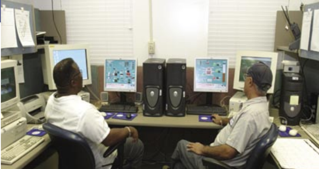
Monitoring operations at the Plum Island Plant using the SCADA system.
