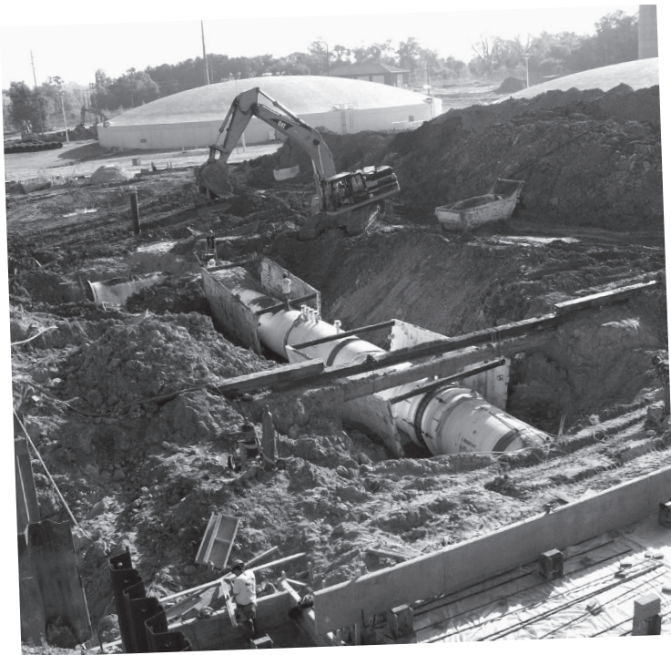
At 7 feet in diameter, this new pipe will enable more water to flow from the filtration basins to storage tanks for disinfection—the final step in the treatment process.
